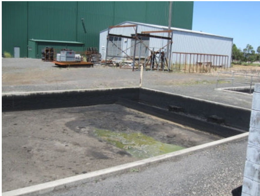
Photograph 6 Triple interceptor pit for fire water run-off
