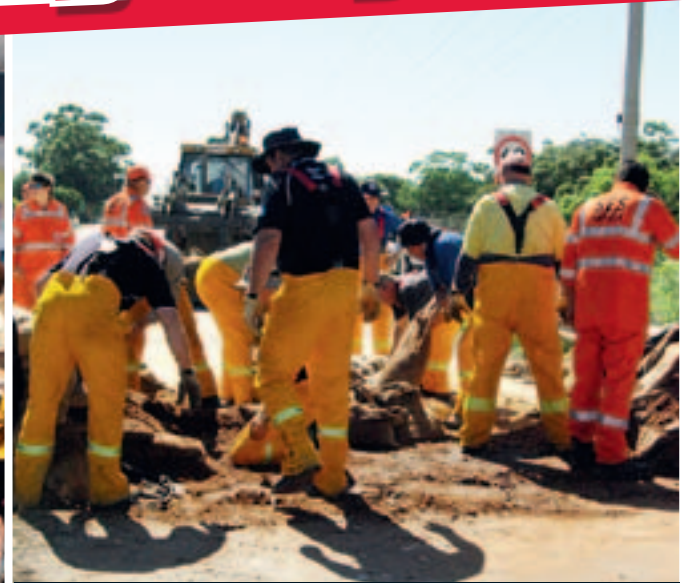
Sandbagging Patchell Bridge over the Loddon River, Kerang. Photo supplied by Andre Brown
