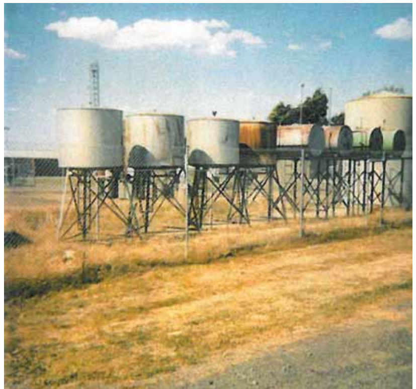
Above ground fuel storage tanks, 1996. Photograph courtesy of CFA
